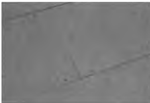
Vinyl Asbestos Floor Tile
