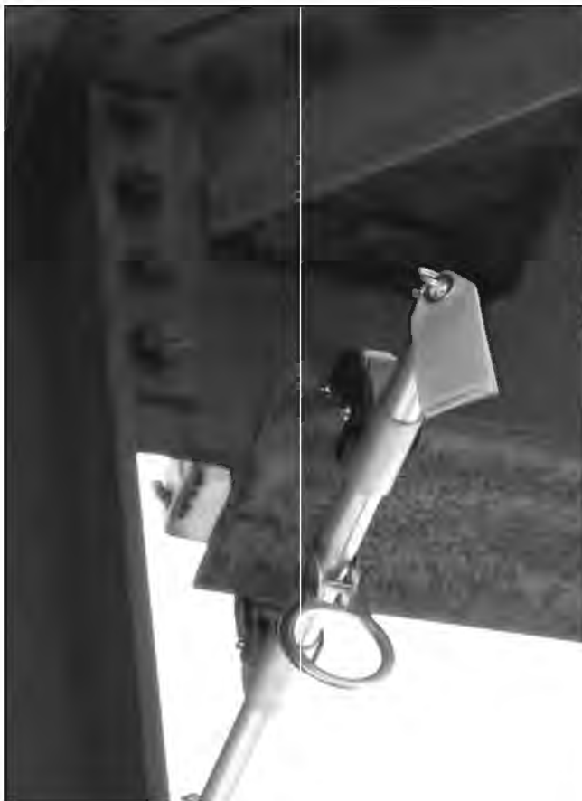
Fig. 16. Danger: Beam clamp near coped end
