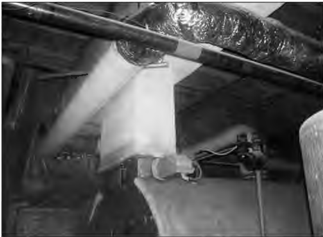
Pipe and boiler insulation
