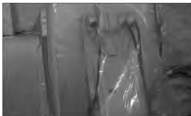
Isolated electrical panel
